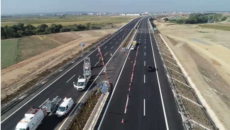
Traffic Management Control
