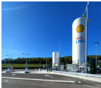
APRR offers two LNG stations in its network
