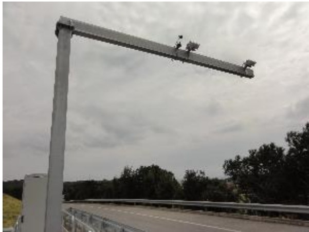
RSU control point
