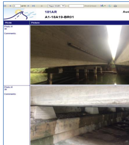
Inspection Reporting Automatically created report
